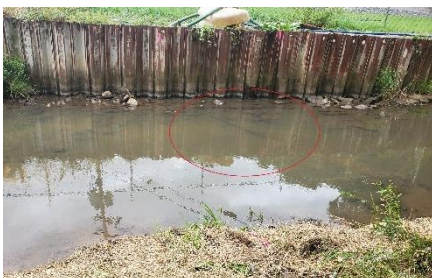
Exposed pipe in stream bank, before.
